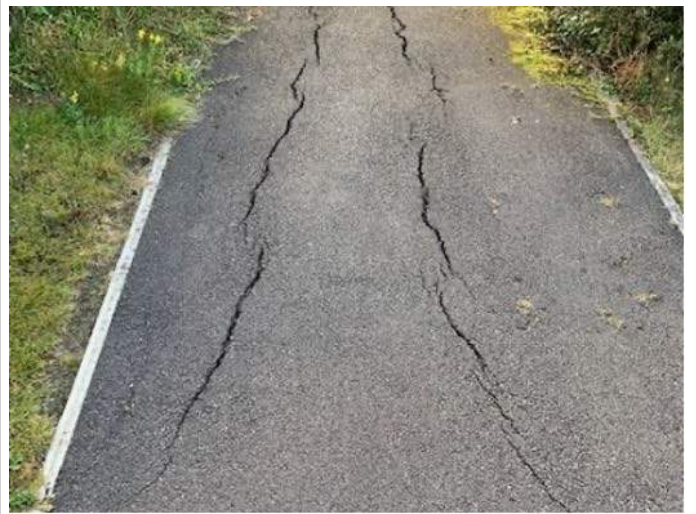
HUNTS GROVE DRIVE - Severe subsidence of path
