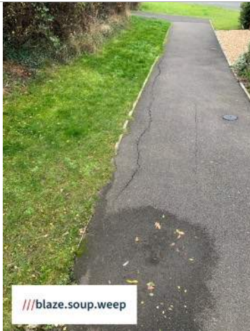
Path Subsidence Hunts Grove Drive
