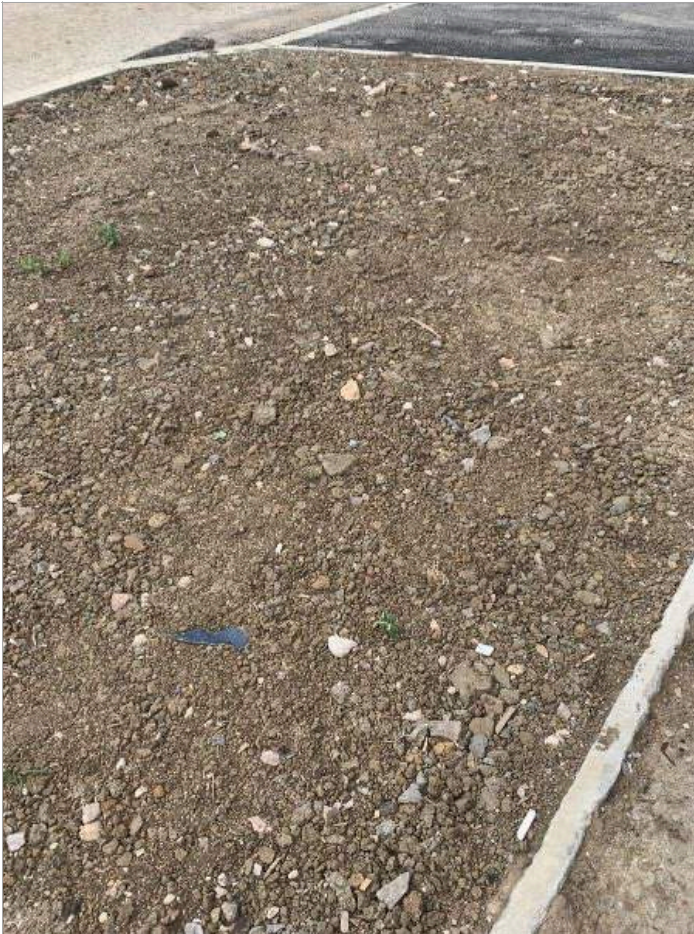
BOVIS - Poor quality of topsoil for verges
