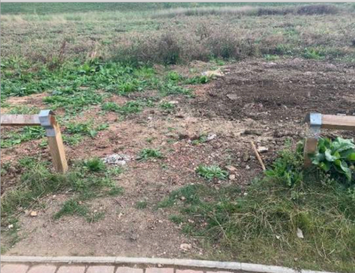
BELLWAY - Missing fence rail and (reported to council) area being used as a dumping ground by resident for building work
