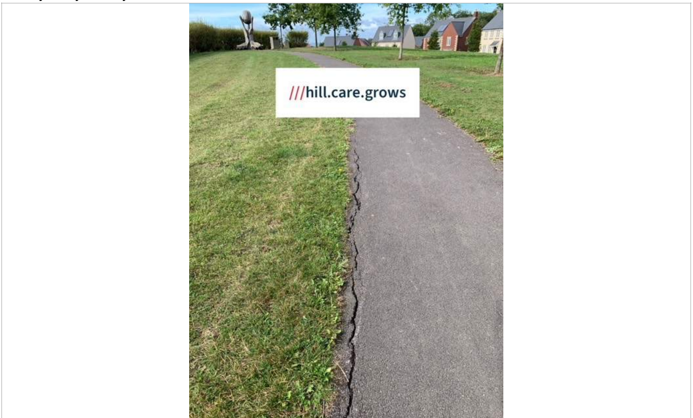
ACORN PARK - path subsidence
