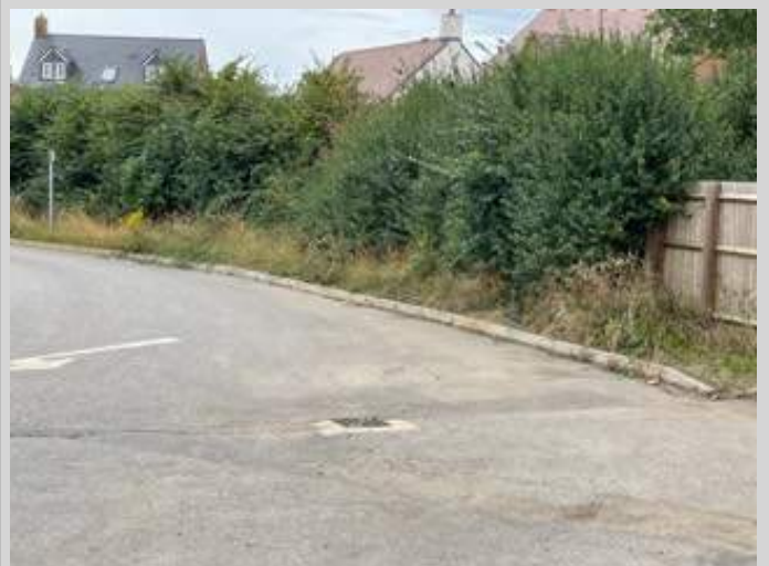
HARRIER WAY - Behind the boarding, the verges and the hedgerow are very overgrown.
