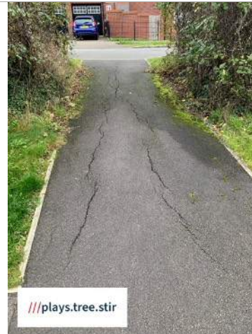
Path subsidence Hunts Grove Drive
