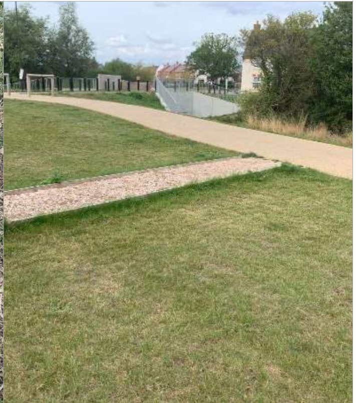
BELLWAY - Temporary path, removal and grass needs restoring properly
