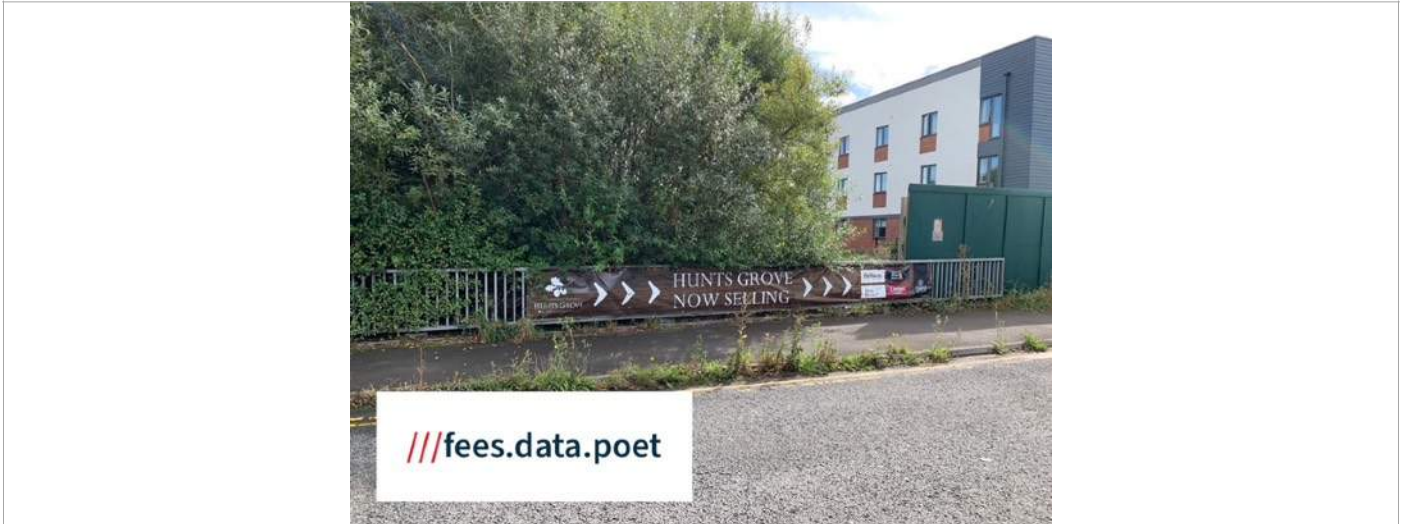
Marconi Drive - Overgrown and substantial weeds in kerb
