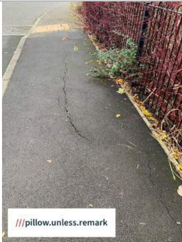
Path subsidence Hunts Grove Drive
