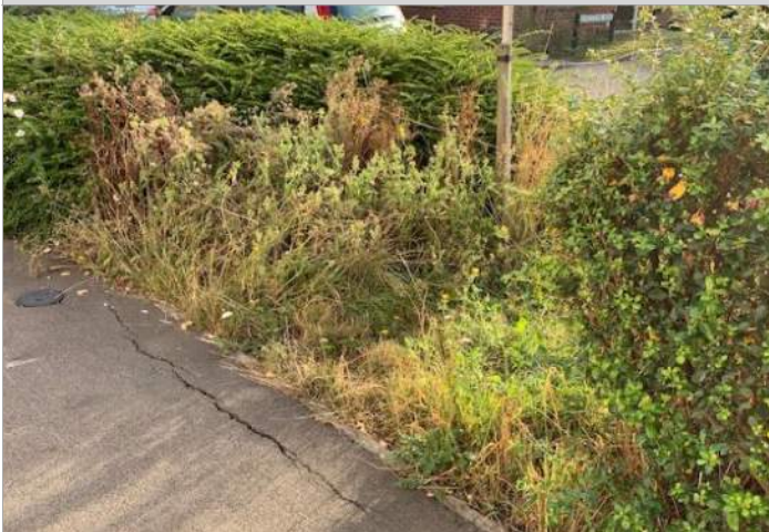
HUNTERS WAY - Weeds in verge and path subsidence
