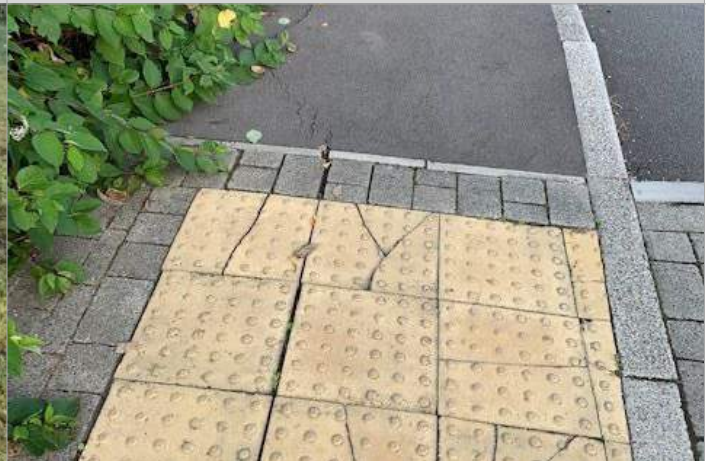
LIME TREE AVENUE - Pavers damaged
