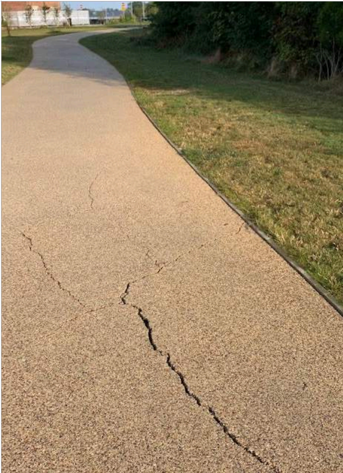
BELLWAY - Massive subsidence along new path between Bellway and Shorn Brook
