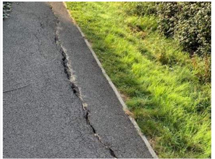
WILLOW EDGE - Pavement subsidence
